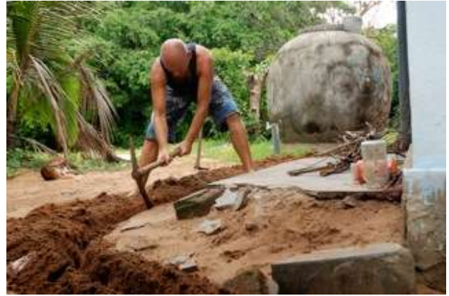
KarunaRathna Water pipeline
